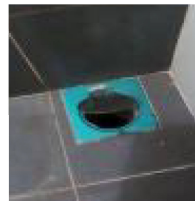
The floor trap cover is bent and cannot be closed, leaving a large gap (P1)
