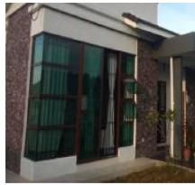
"The sliding door is not covered with shade, at the front of the house. The rainwater easily enters the house." (P2)
