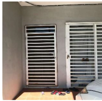
"The main door is beside the sliding door. So, if I accidentally left my keys in the house, I could just jerk the sliding door's lockset and open the main door easily. So, it shows lack of safety for the design". (P6)
