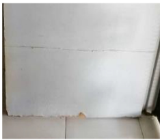
"...the rainwater penetrates through windows - two rooms at the back affected... the roof eave is insufficient; the rainwater hits the main door directly. So, the timber door got damaged." (P3)
