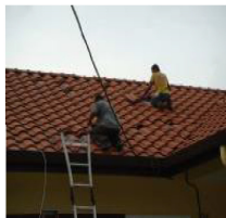
"The height and narrow space between the roof and ceiling caused the electrician to work from top of the roof for wiring purpose. That's dangerous." (P5) * Picture by P5
