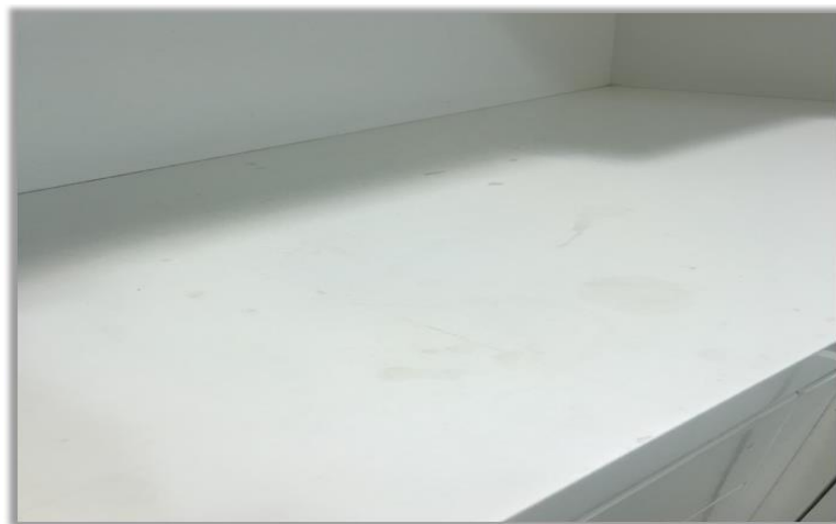
Figure 7.27 Stains in Kitchen 2 (Source: Author)
