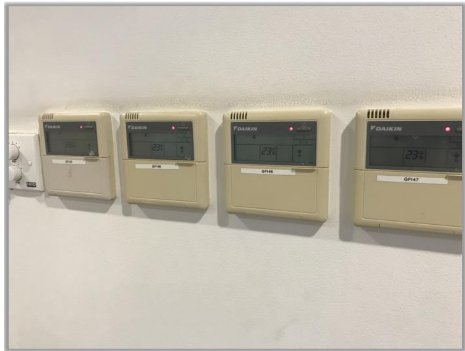
Figure 7.28 AC Control (Source: Author)
