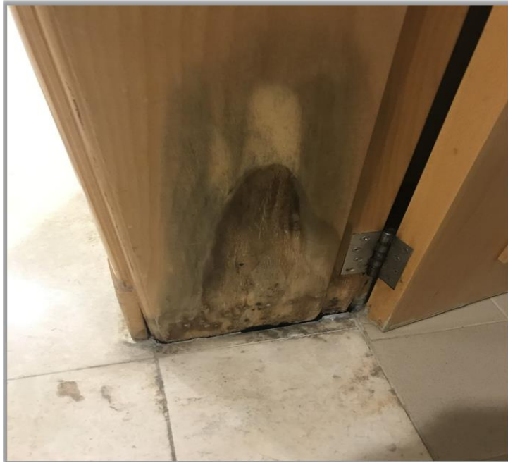
Figure 7.23 Wooden Door for Toilets (Source: Author)
