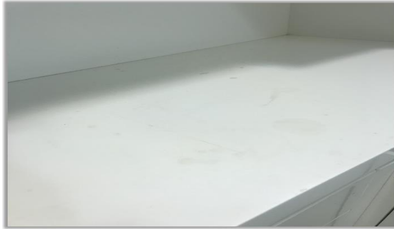
Figure 7.26 Stains in Kitchen 1 (Source: Author)
