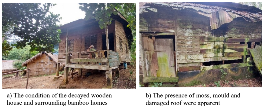
Figure 5: The condition of a wooden house initiative by the government in Jerai 1 Village
