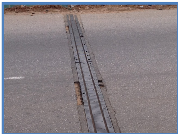
Figure 3a. Deteriorating expansion joint
