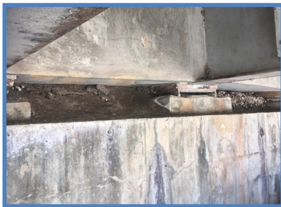
Figure 17. Soil loss from roadway approach. Source: Field Survey 2019
