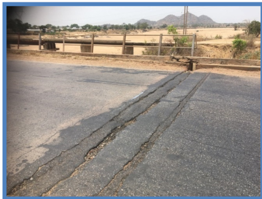
Figure 19. Spalling on approach joint.
