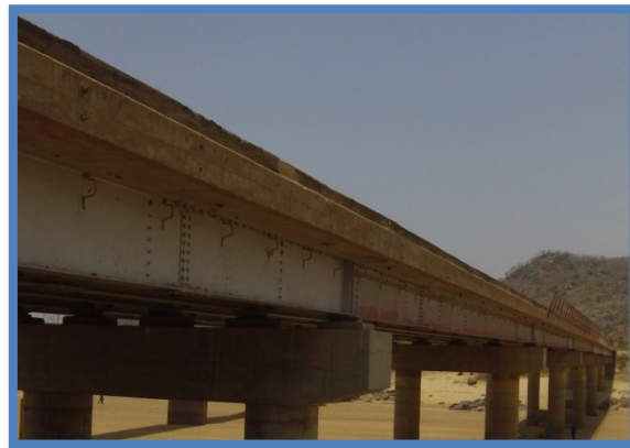
Figure 20. Missing railings due to vandalism.
