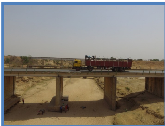
Figure 22. Noticeable absence of railings.
