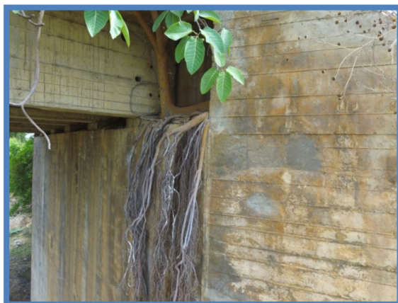
Figure 7. Tree growing on abutment seat. Source: Field Survey 2019
