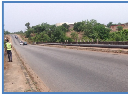
Figure 13. Missing railings due to vandalism
