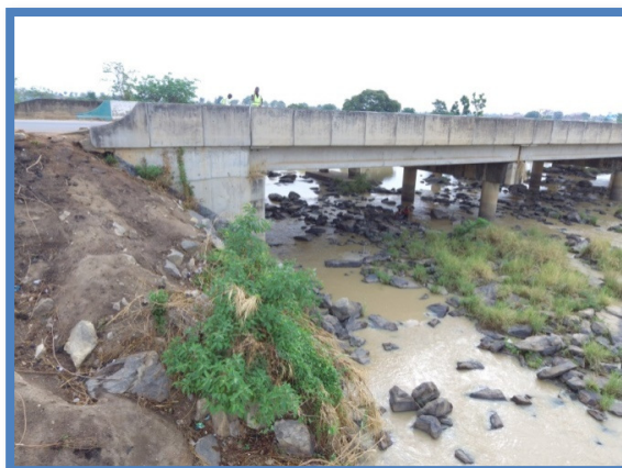
Figure 4. Dislodged stone pitching Source: Field Survey 2019
