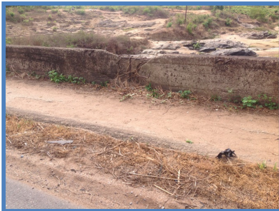
Figure 9. Major spalling of crash barrier Source: Field Survey 2019
