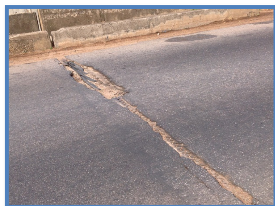
Figure 3b. Deteriorating expansion joint.
