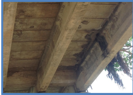
Figure 12. Blocked drain and tree growth. Source: Field Survey 2019
