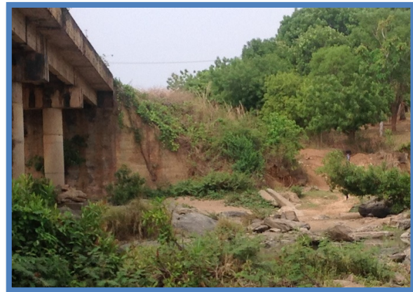
Figure 10. Unwanted vegetation on embankment.
