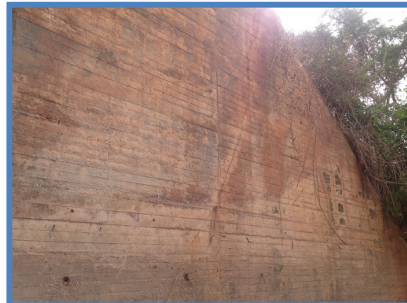
Figure 8. Pronounced crack on wing wall.
