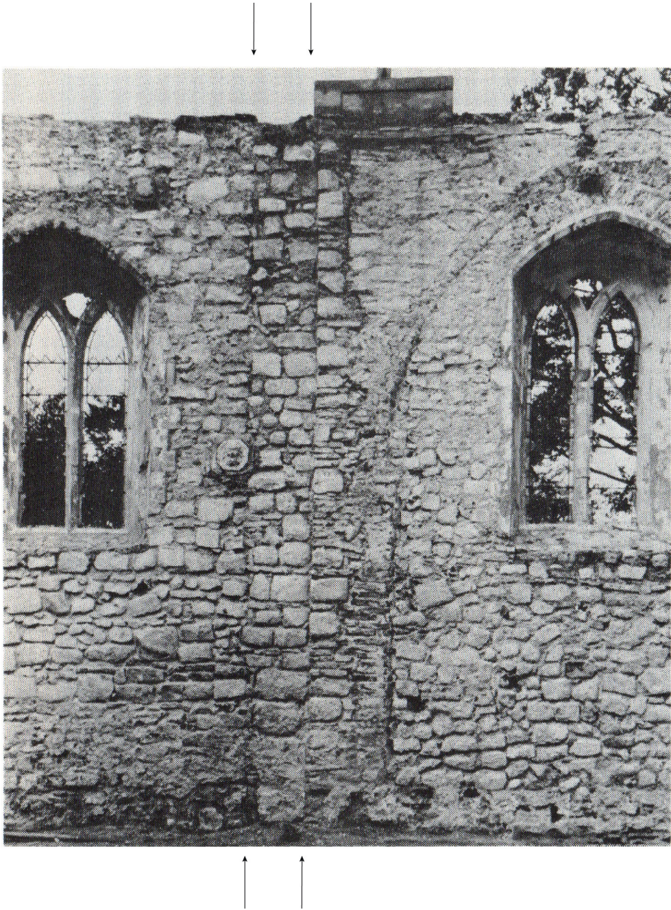
Figure 19. Interior view of the north wall of the nave (Rose 1994, pl. 1A, reproduced by kind permission of the British Archaeological Association). The arrows indicate the vertical joints in the nave wall.
