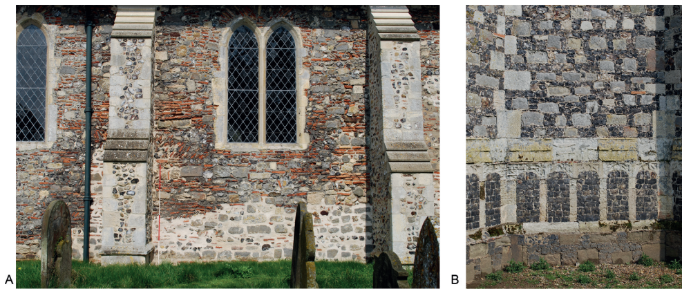
Figure 4. St John the Baptist, Reedham: (A) south wall of the nave with a mix of grey quartzite and Roman brick and tile; (B) south side of the tower, grey quartzite blocks and flint.
