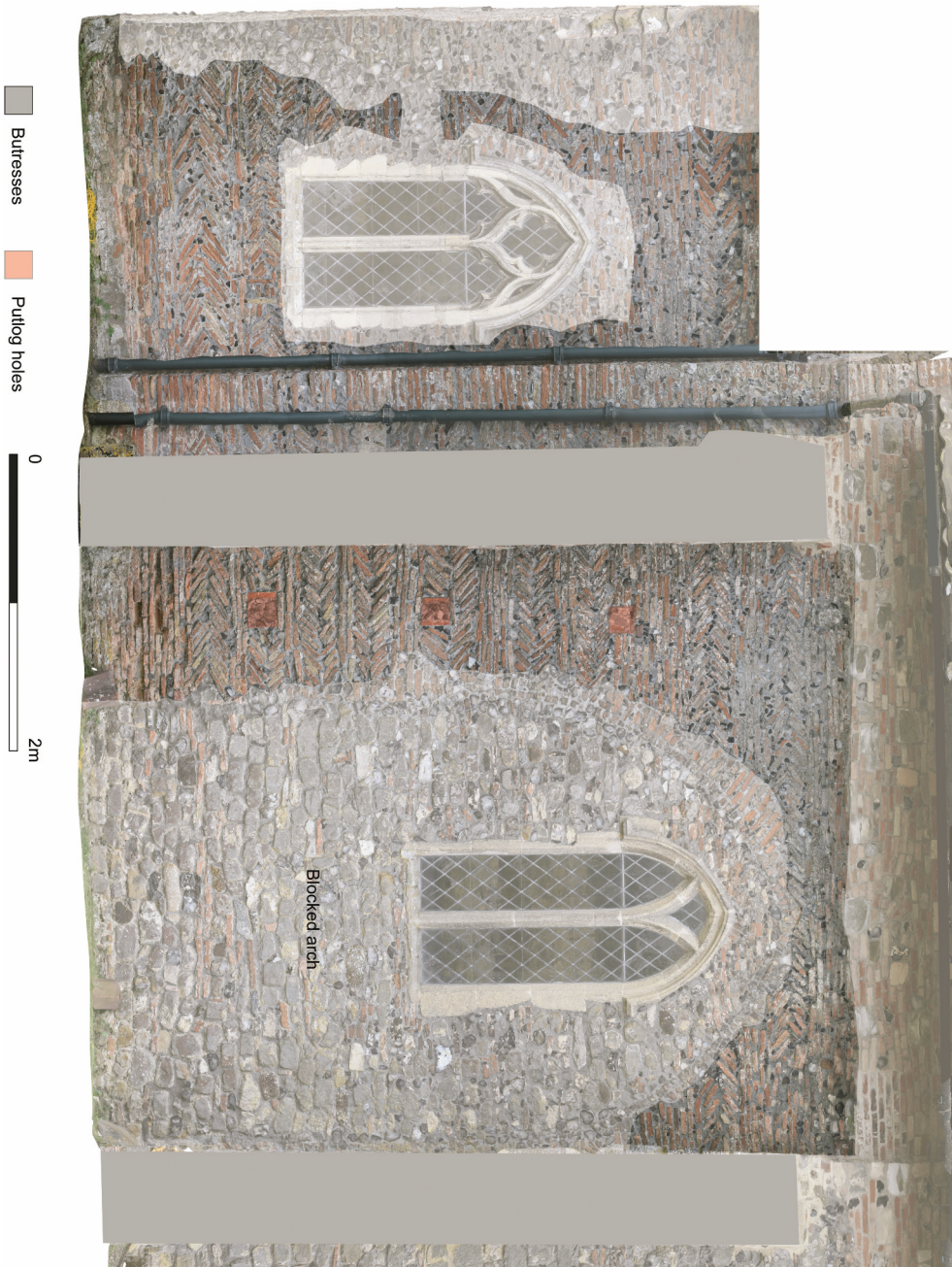
Figure 20. Rectified photograph of the brick-built north wall of the nave with the later, blocked arch highlighted.
