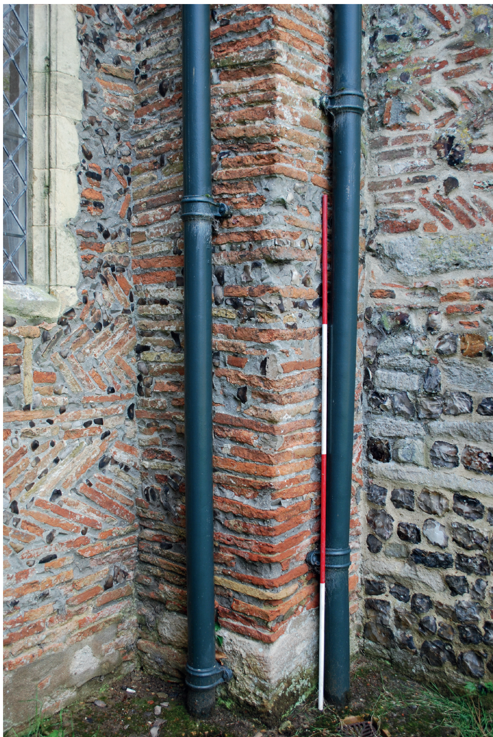
Figure 17. North-east corner of nave with quoining of re-used Roman brick and tile.
