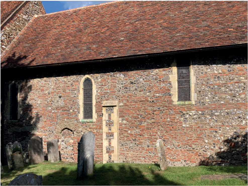
Figure 22. The north wall of the chancel, originally the nave, of St Martin's, Canterbury.
