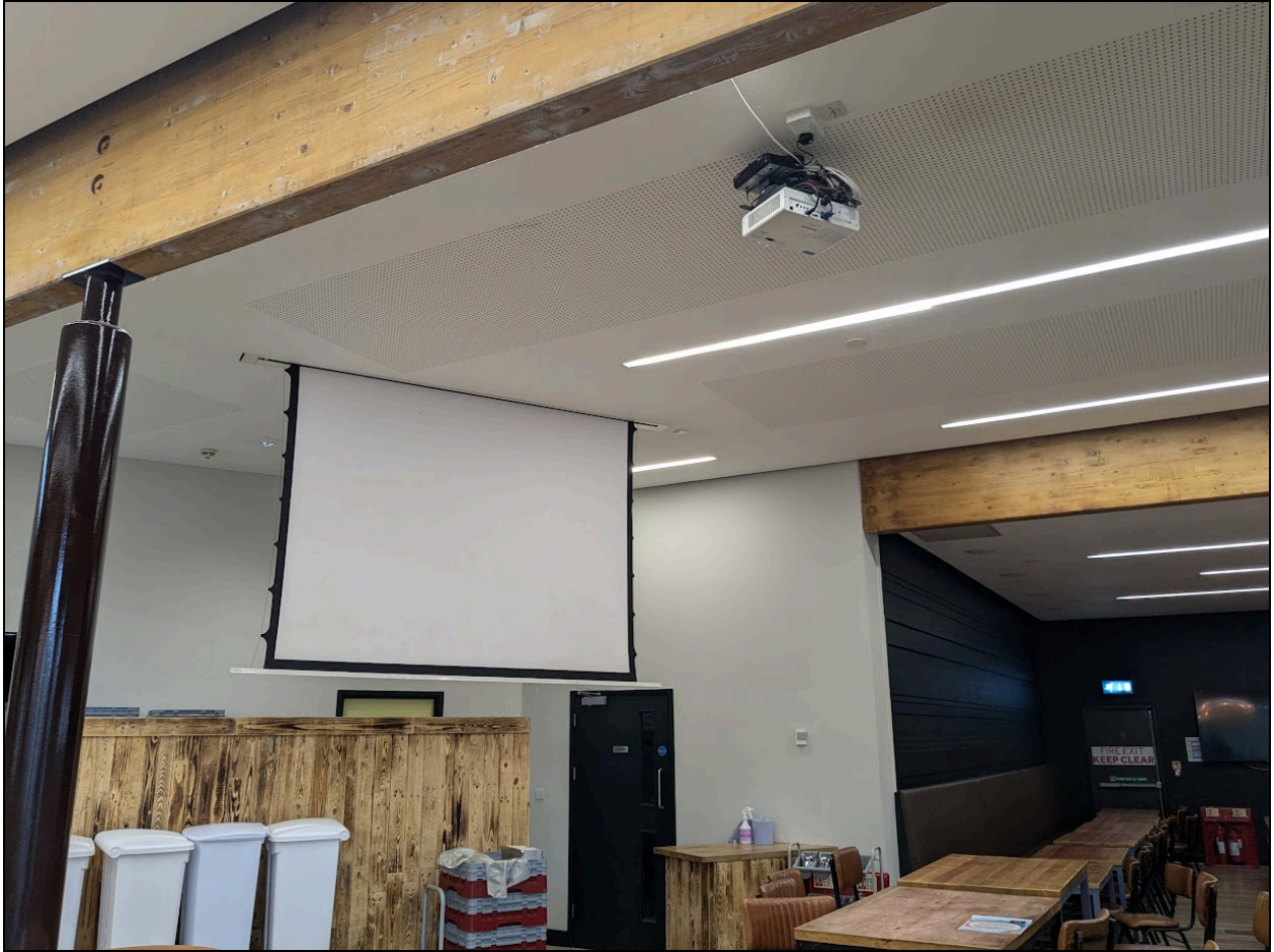
Figure 17. Front of the house DG2-100-0-493 socket and projector
