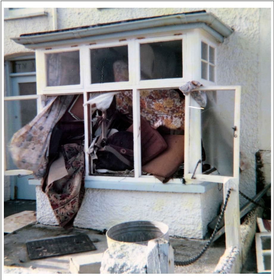
Figure 6. Storm damage to Ty Haf , January 1976.
