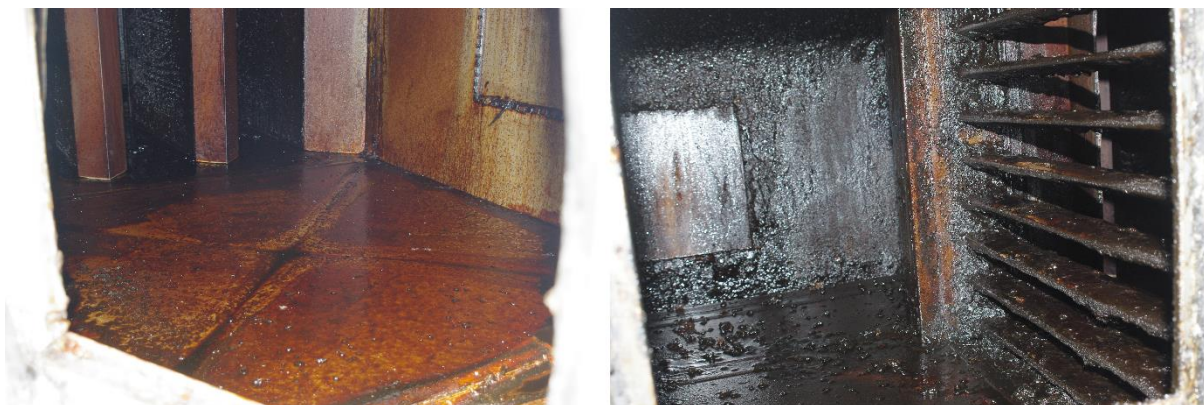
Figure 3: Trial site ventilation duct interior 3 weeks post manual duct clean
