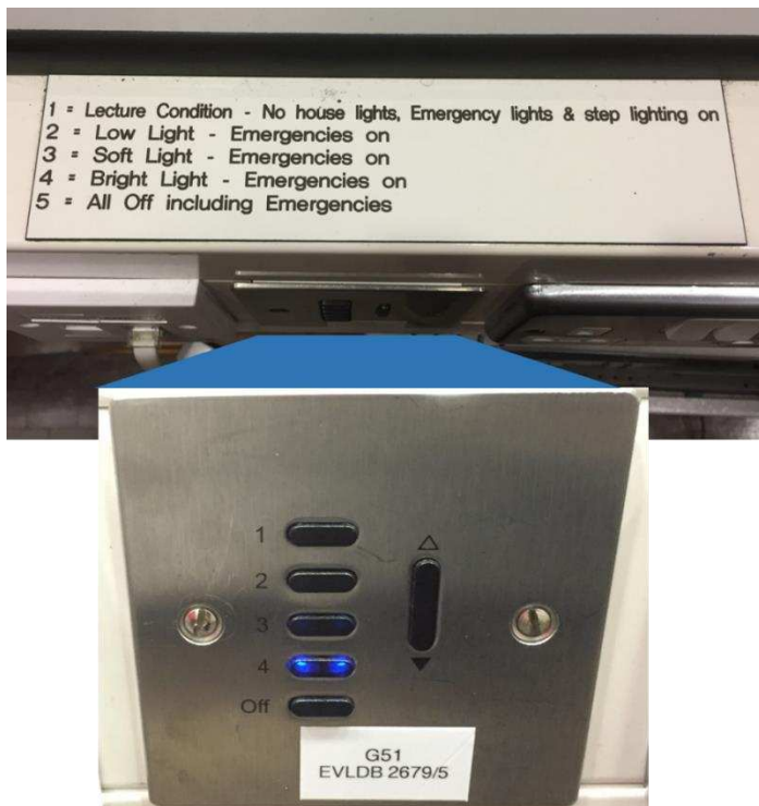
Figure 2. Chemistry lecture theatre light switch
