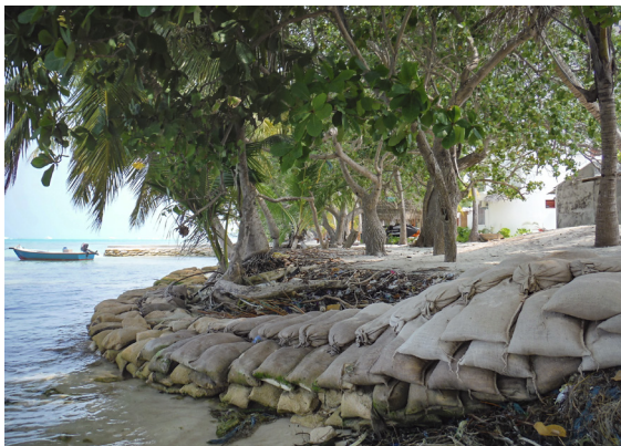
Cover photo: Sandbags piled up to slow down coastal erosion. © Alex Arnall.
